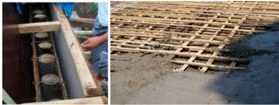
Figure 8: Bamboo that is woven and placed horizontally is then concreted. b) Bamboo rods are used instead of concrete reinforcement for columns (Hildayanti and Wasilah, 2023)
