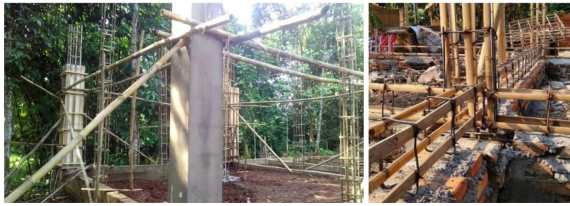
Figure 7: Bamboo rods instead of concrete reinforcement in columns (Hildayanti and Wasilah, 2023)
